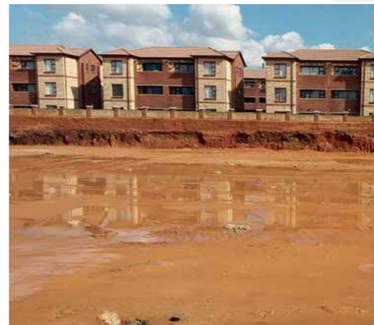
In April over 100mm of rain caused severe flooding of the basement works which required two days to pump dry
